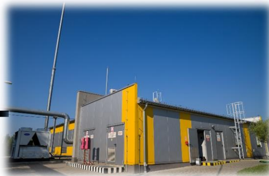
Methane-reduced demethanation system. Drainage station
